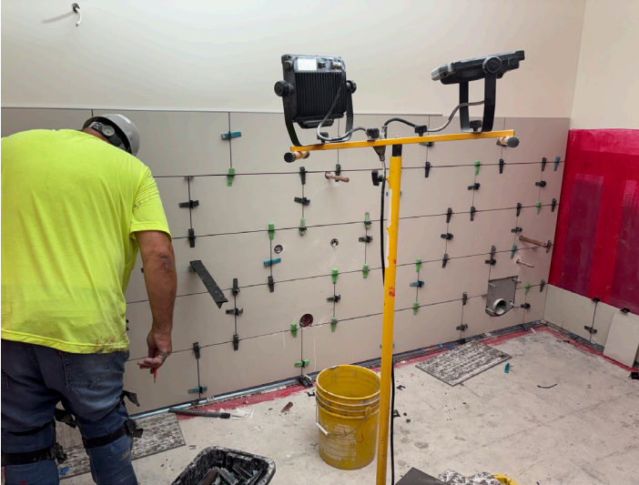
Floor & Home installing the tile within the lobby bathrooms in Area A.
