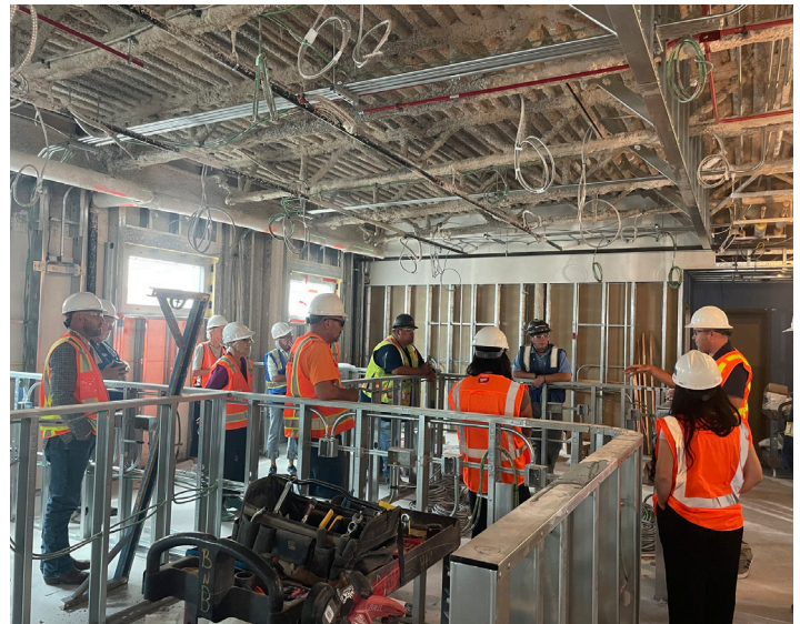
Bouten assisted In leading a tour throughout the facility on August 6 to show the current progress of construction.
